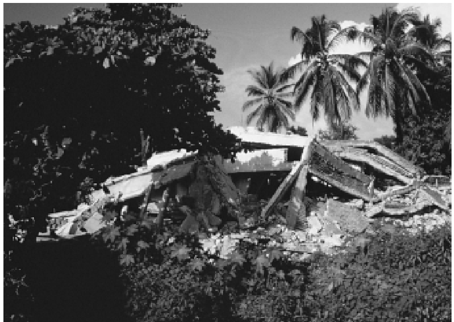
Residence that collapsed on access road to Costa Real Hotel, Manzanillo, Mexico
